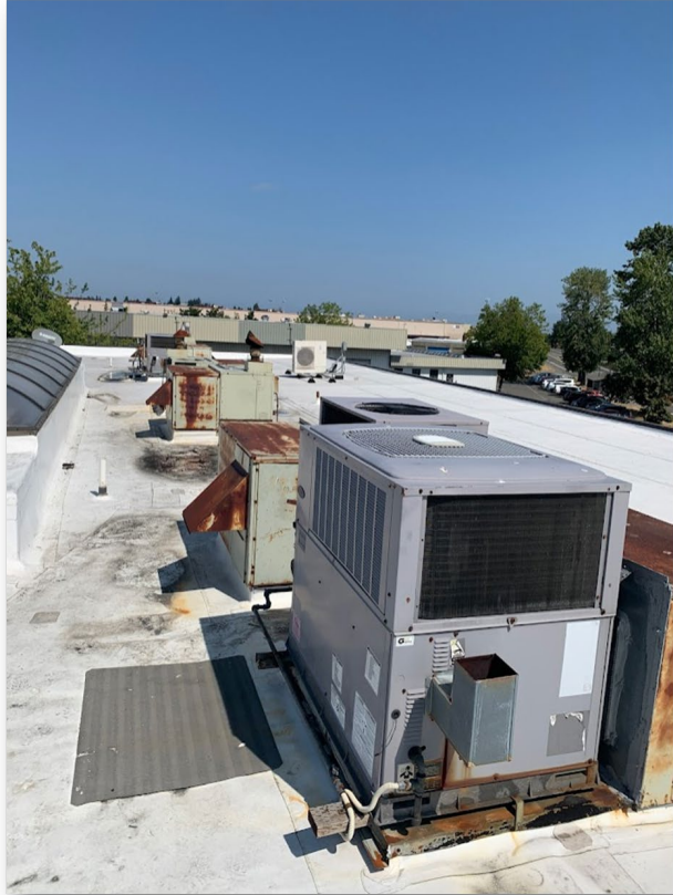
HVAC units & air handlers
